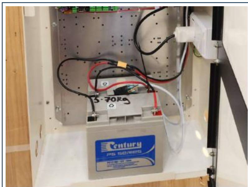
Figure 7: Front-to-back 18Ah batteries installation
