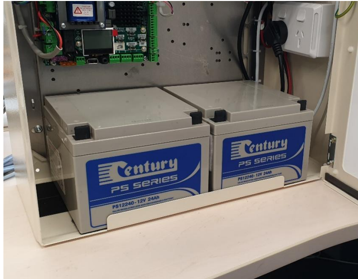
Figure 5: The two batteries successfully installed
