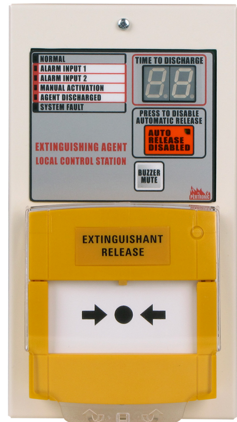
Local Control Station (LCS)
